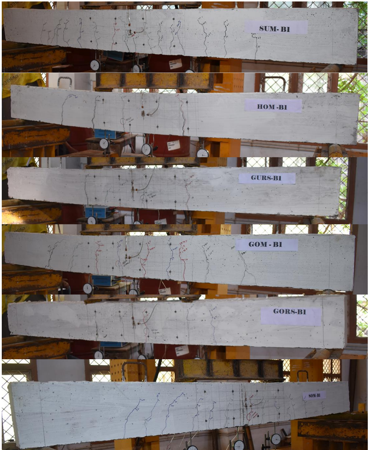
Figure 9: Failure of beams
