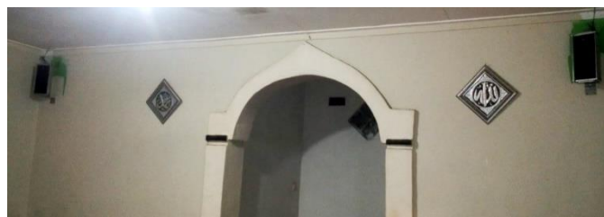
Pic 12. Speaker has been installed for room acoustic system
