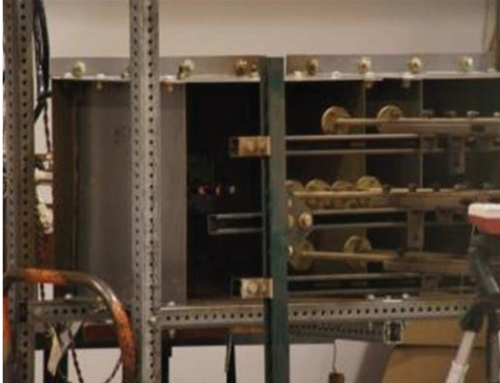
3. VCBB -Vertical conductors/electrodes terminated in an insulating barrier inside a metal box/enclosure.
