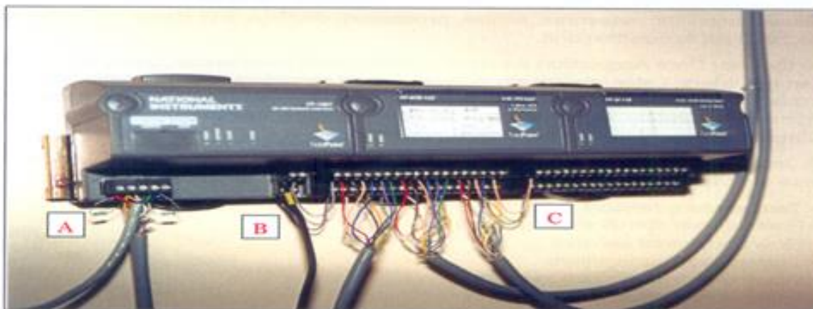
Figure 1 Field point network node in the office of SEES building.
