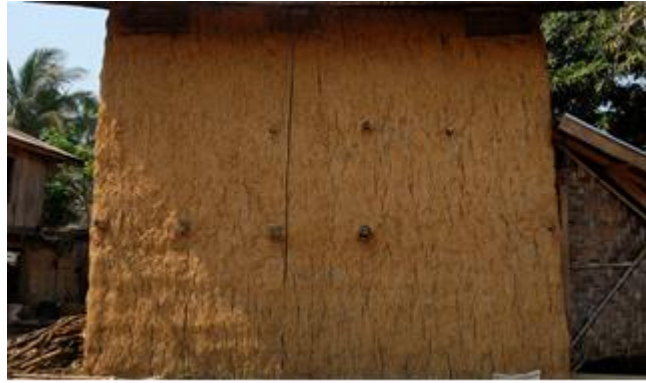
Figure 11 a straw and grass mixed with clay for the wall of tobacco kiln
