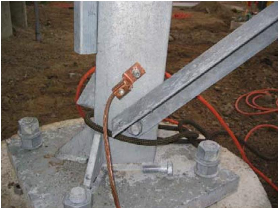
Figure.2: A tower with a heavy copper ground wire
