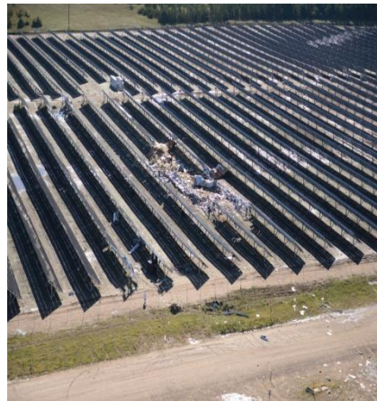
Figure 1. Camp Ripley received damage 60 acre solar field, during a big storm and tornado Sept 7, 2016.
