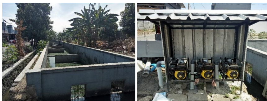
Figure 2. Retention Pond And Pumps At De Marrakesh Residential
