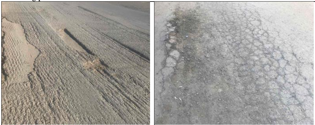
Figure 6: Represents cracks and potholes on the road in the city of Al-Khalidiya
