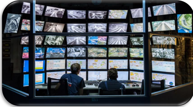
Figure-4: Control Room for Traffic Congestion and Road Surveillance
