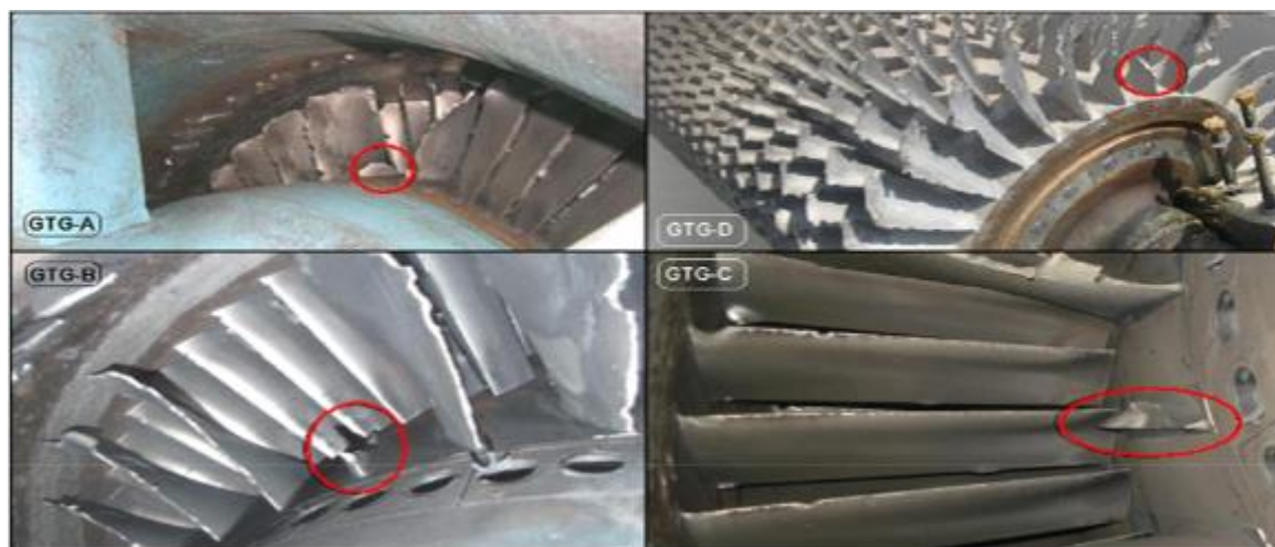
Fig. 1 Failed blades in first row of four frame-6 gas turbines
