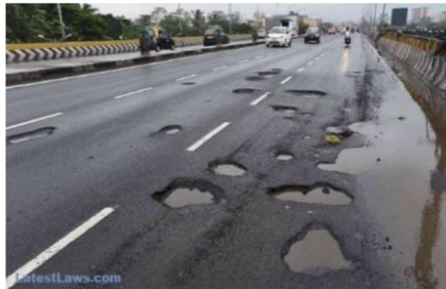
Fig.6.A - Test image of potholes
