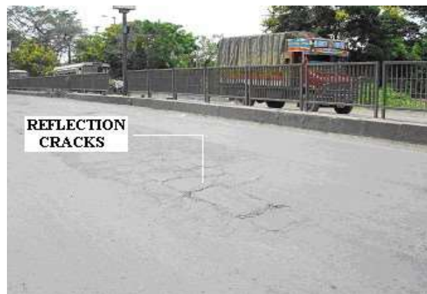
Figure 1. Reflection cracks on overlays with further weakening due to propulsion of secondary cracking
