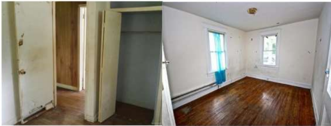
Figure 5 a: Room condition is critical, door damage critical, floor damage is major, b: Room condition is major, wall scuff moderate, floor damage major.
