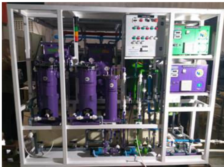
Fig.3 Experimental Set-up of ETD Plant
